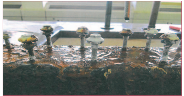
Above: Fasteners sold in South Africa as Class 4 tested by SABS failed dismally in salt spray test.
